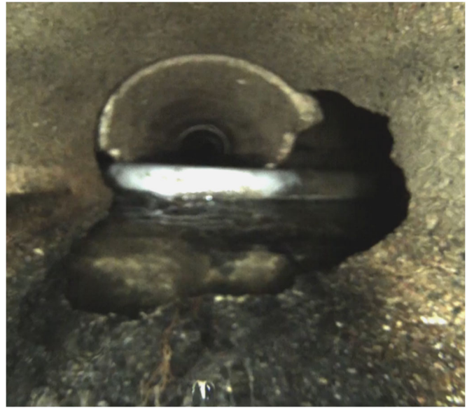
Picture shows a telecommunication cable going through a sewer pipe. Found during regular TV inspection.
